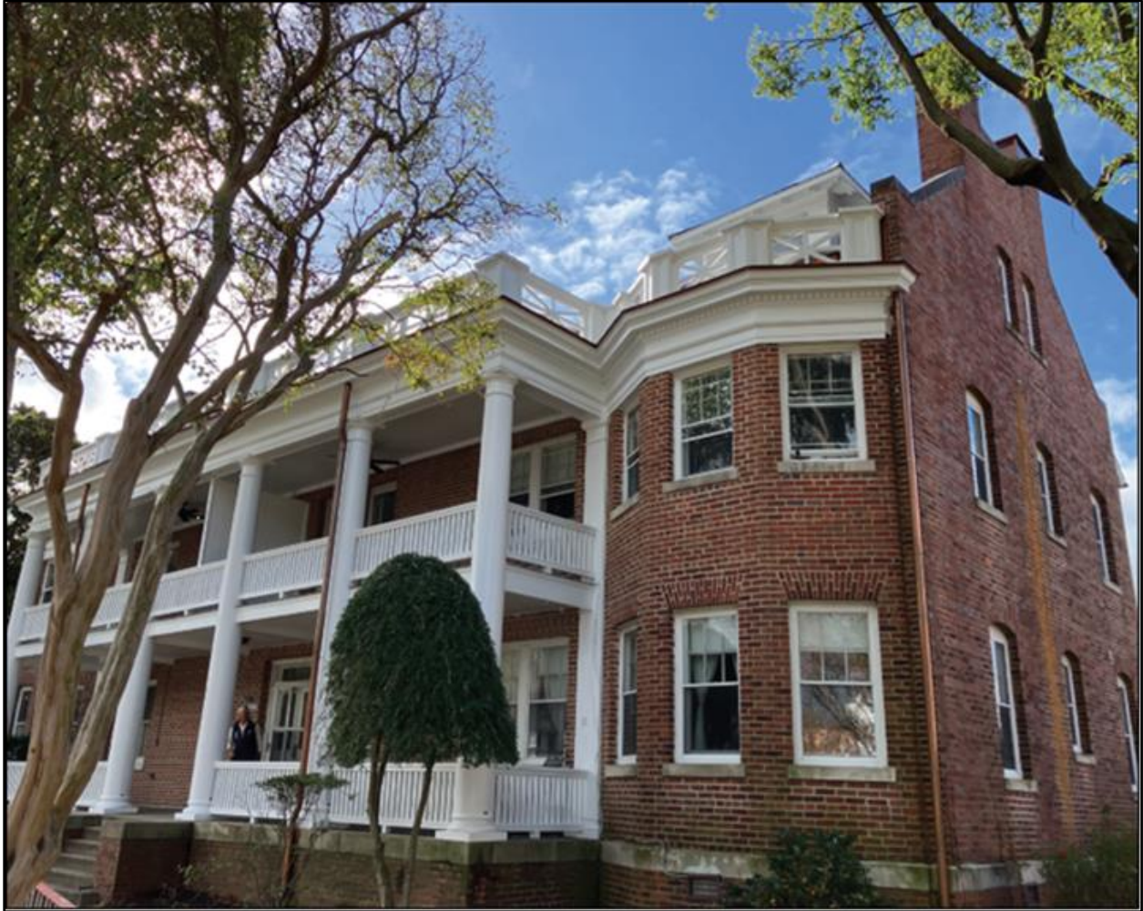
Image showing Building 143 with restored front porch or loggia as well as rooftop balustrade
